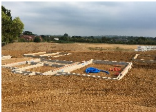
House building in the parish began in earnest in the summer of 2016 and work is now underway on at least 5 sites across the parish.
