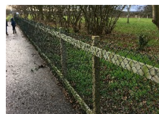
New fencing at Deardon Field which is managed by Shinfield Parish Council as an open recreation space and community orchard, located off Deardon Way
