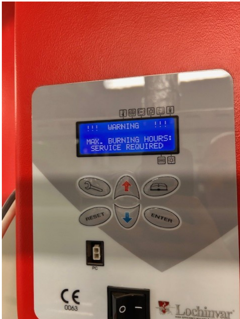
Water heaters : Service Required
