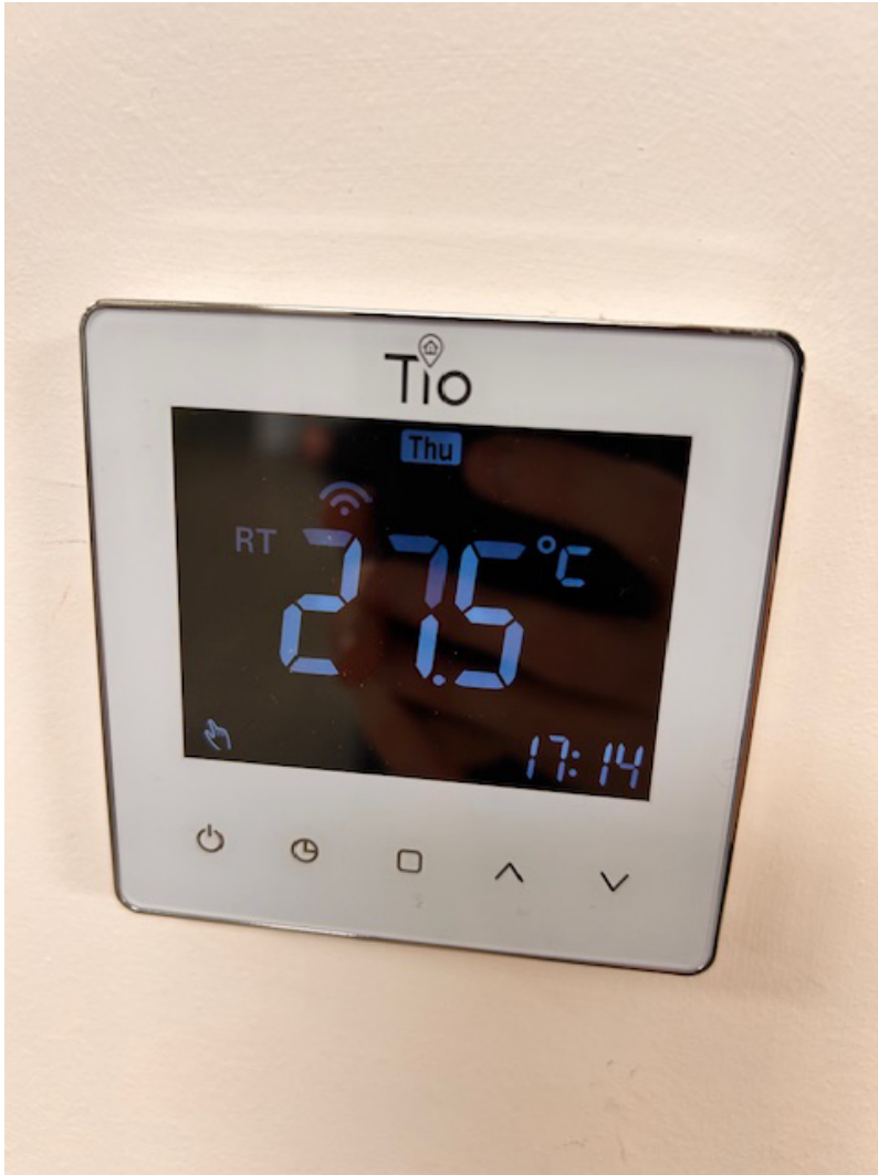
Underfloor heating programmer : note temperature setting !!!!
