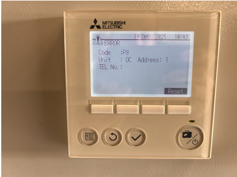
Error code on main ASHP's, reset and programme heating flow temp.
