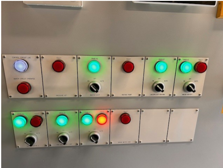
Plant observed 'on' (manual) mode. Changed to Auto.
