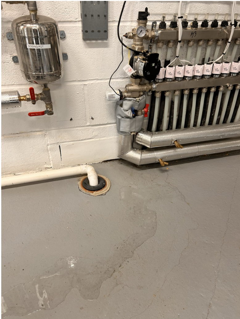
Leaking underfloor heating manifold – non performance
