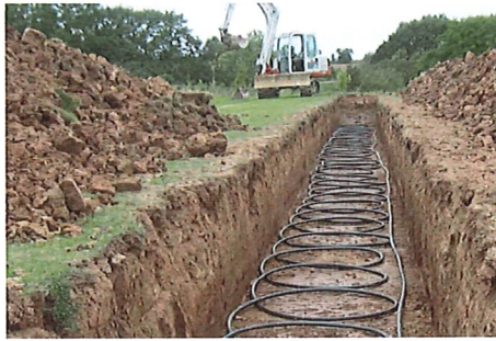
Ground source heat pump 'slinky'.
