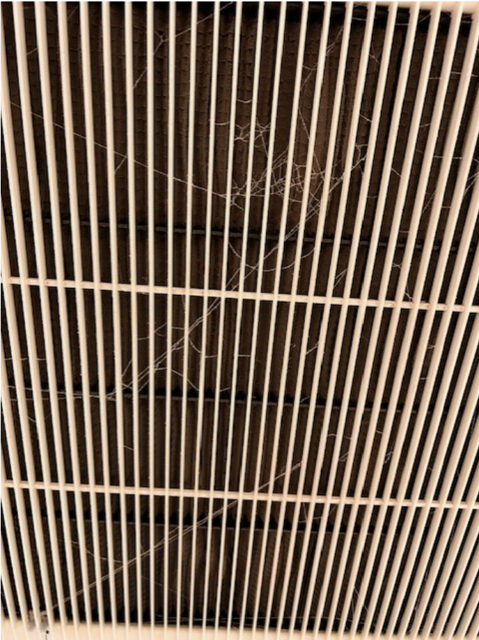
A/C filters in need of clean / filter change.
