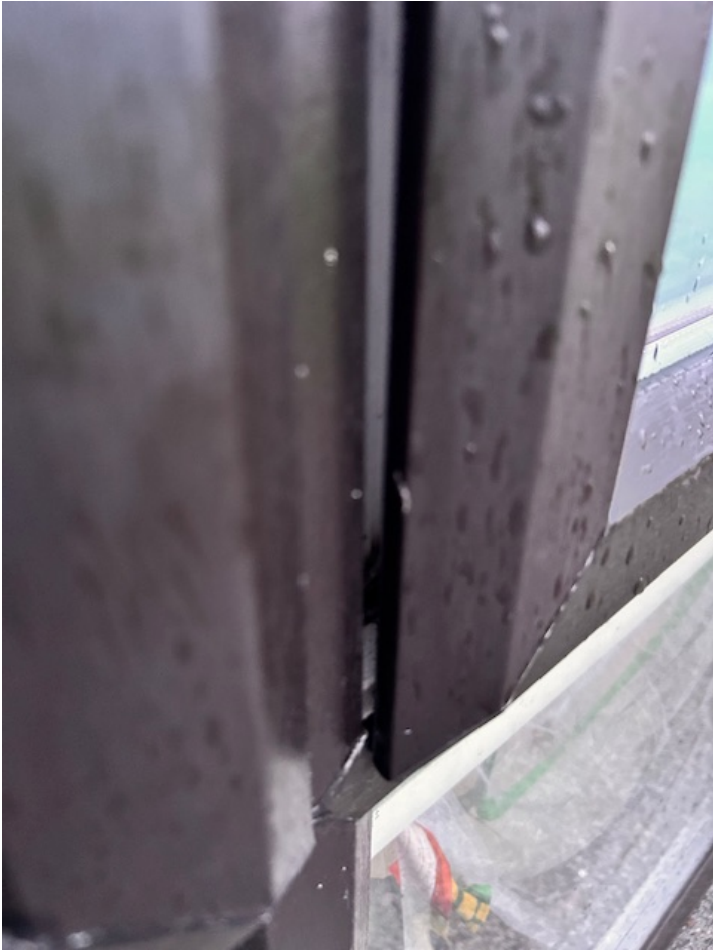
Broken window – repair.
