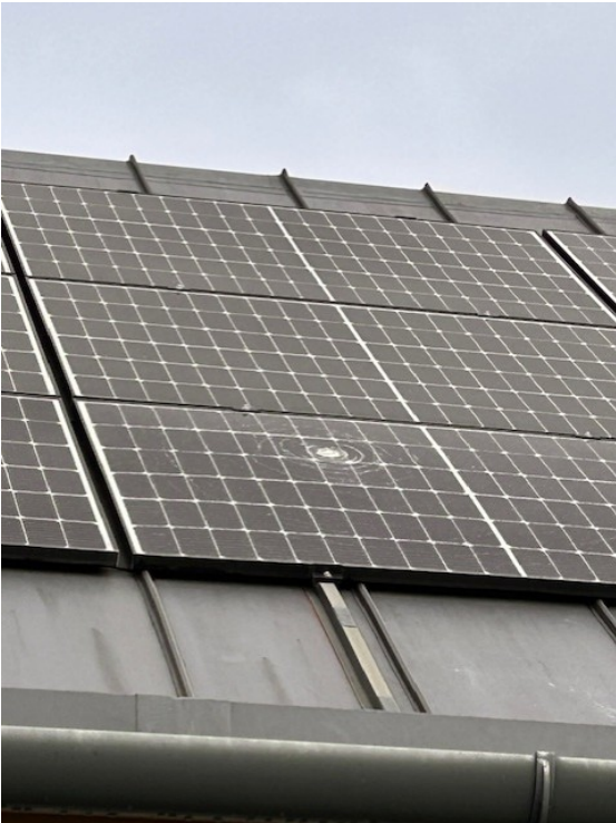
Cricket ball damage to solar PV panels
