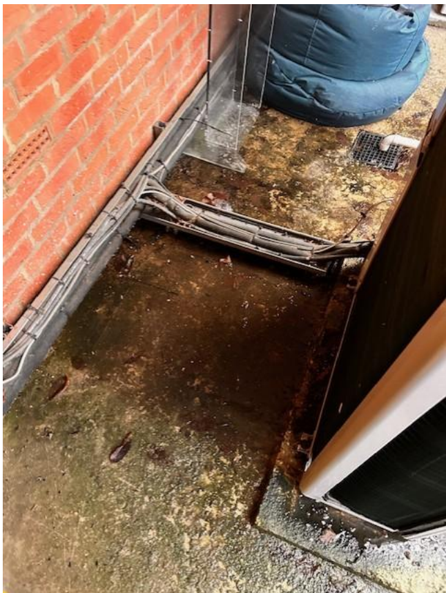
Maintenance Issue – ASHP 'condensing' and leaking.
