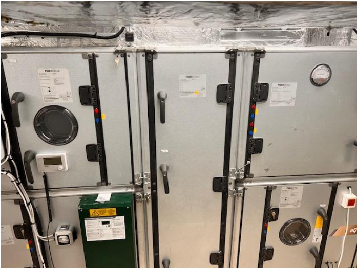
Main heat / vent plant – display not functioning properly.
