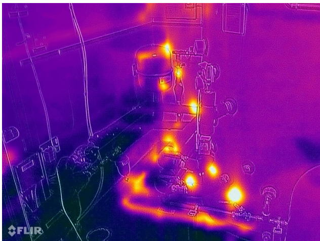
Thermal image of heat loss due to uninsulated pipes and valves
